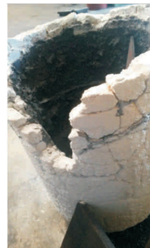
Figure I Cracking as the result of the lining hanging up
